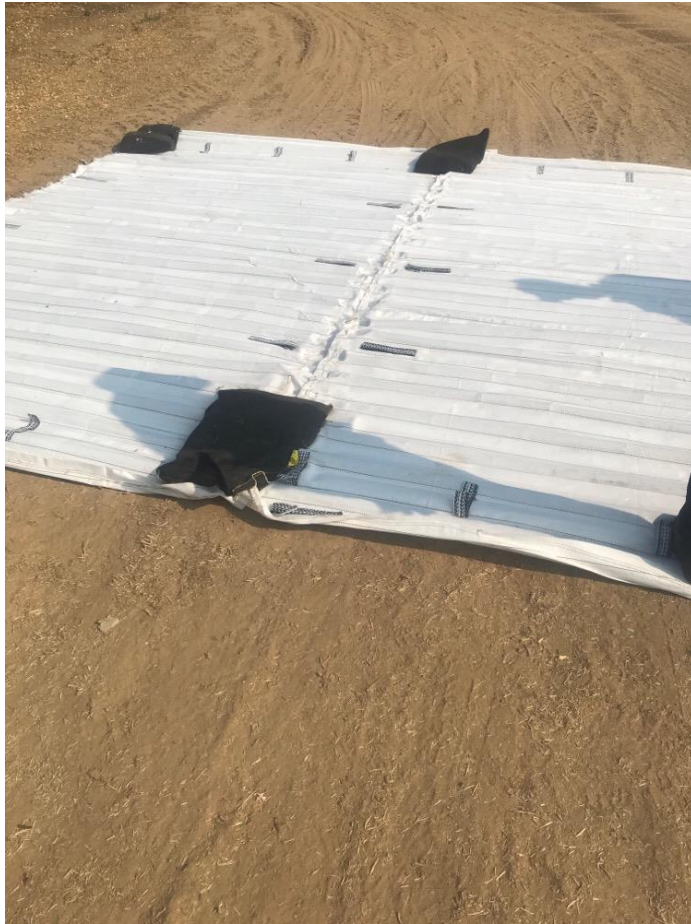
Photo 3: Portable rumble strips to prevent track out in place near Pole 3/31 in accordance with APM HYD-1.
